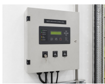
Demo control panel
