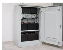
Demo battery backup
